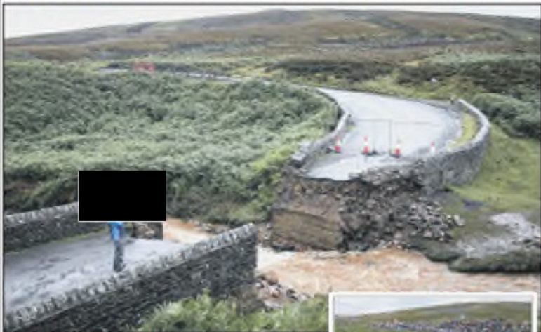
TOBERNICE: The bridge at Capheaton Hill, on Great Wharfe in Tobernice, which was on the route of the 2014 Tour de France, right, was swept away in the storm.
